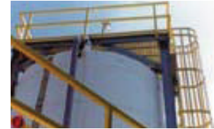
Tanks, grating and railing systems
