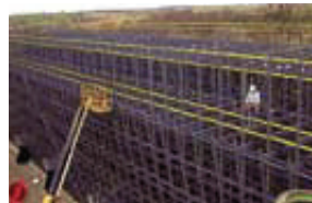
Cooling towers in power plants
