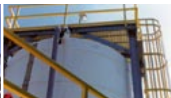
Tanks, Grating and Railing Systems
